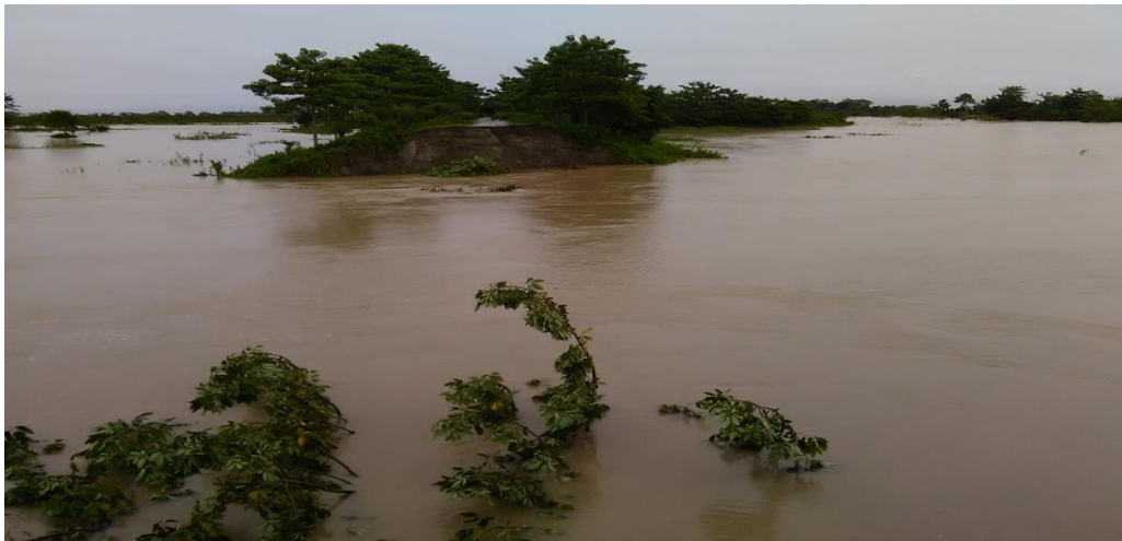
PLATE 1: A View of the Damaged Embankment After Breach or Erosion
